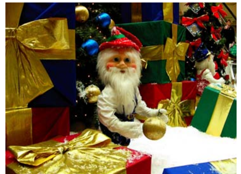
Don't cover transformers with presents or decorations. This is a common cause of fires at Christmas.
